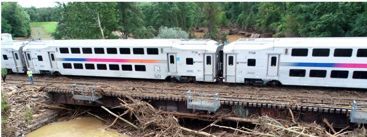
Flood damage to NJ TRANSIT tracks and rail bridge
