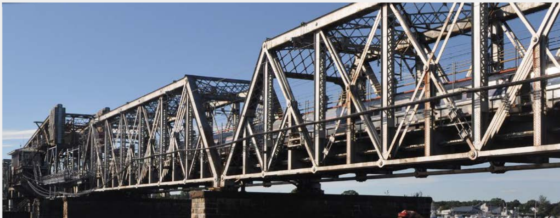
The Connecticut River Bridge Replacement Project is part of the Brook Project Group
