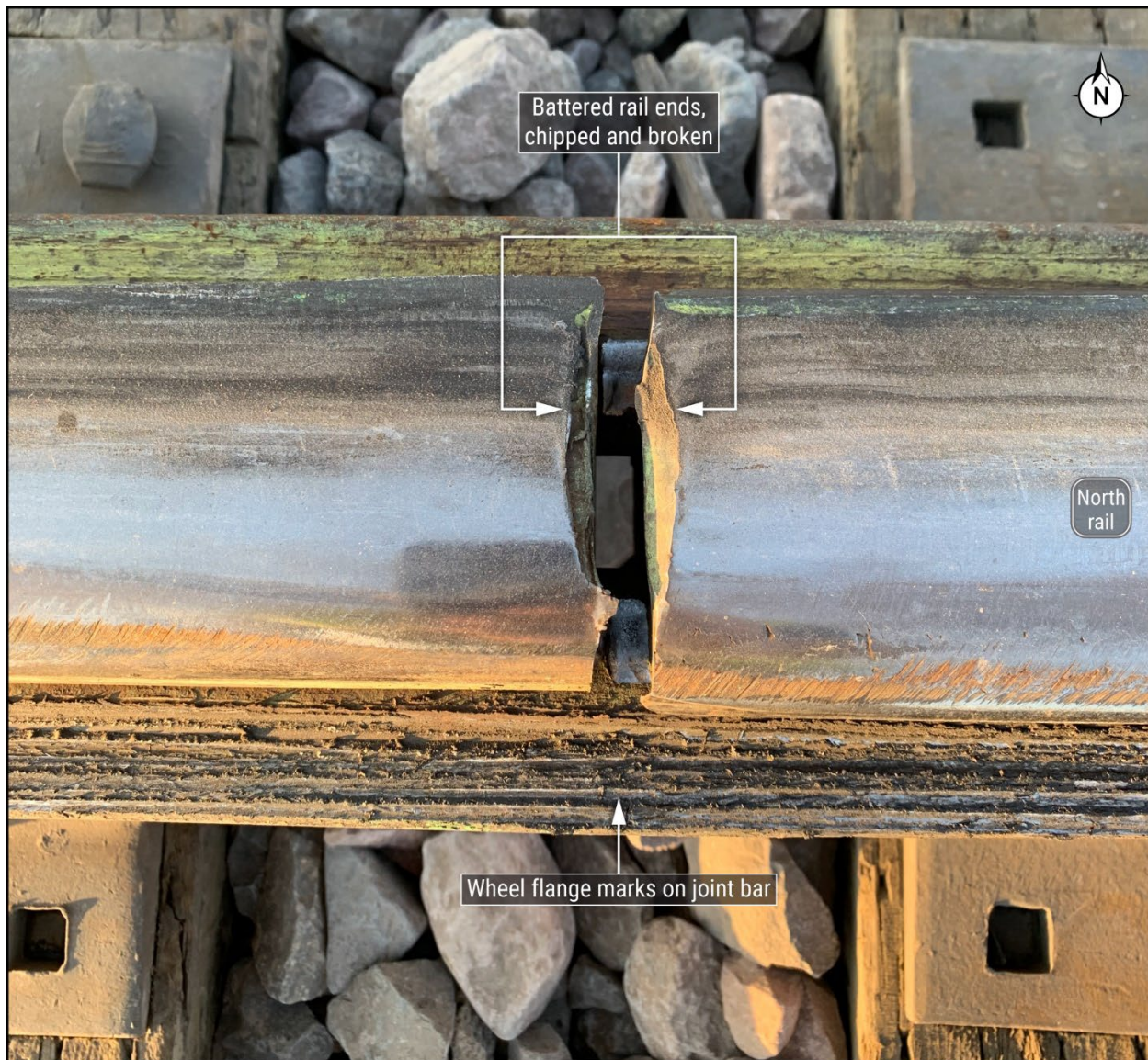
Figure 17. Photograph of the four-bolt rail joint with wheel flange contact on the joint bar. The top of this photograph shows the battered rail ends.
