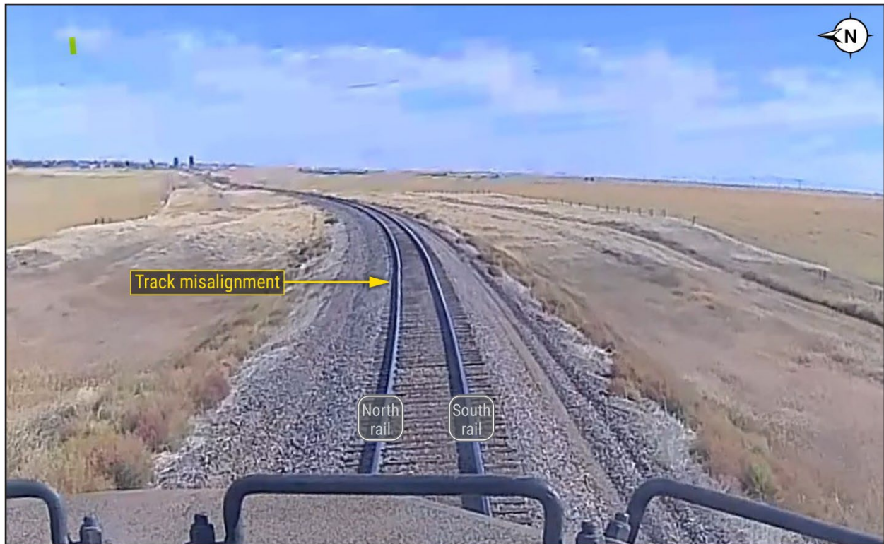
Figure 5. Still frame from BNSF freight train 4182-ZSSECH-24A that shows the misaligned BNSF track.
