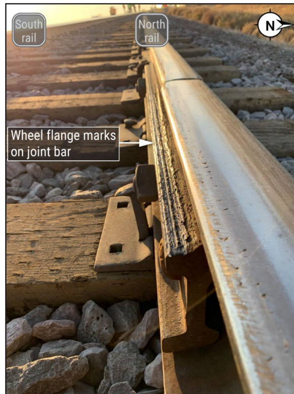
Figure 16. Photograph showing a north four-bolt rail joint with wheel flange contact on the joint bar.
