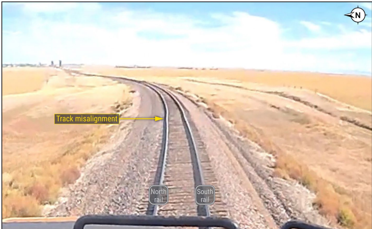
Figure 6. Still frame from BNSF freight train 7380-OPTLCHC3-23A that shows the misaligned BNSF track.
