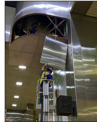
Jefferson Station Ventilation
