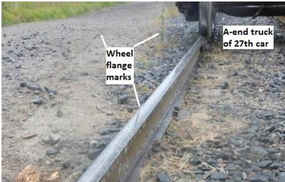
Figure 11. Wheel flange marks on rail head and ballast (Source: TSB)
