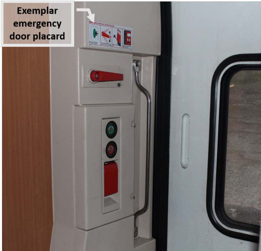
Figure 37. Exemplar emergency door showing instruction placard.
