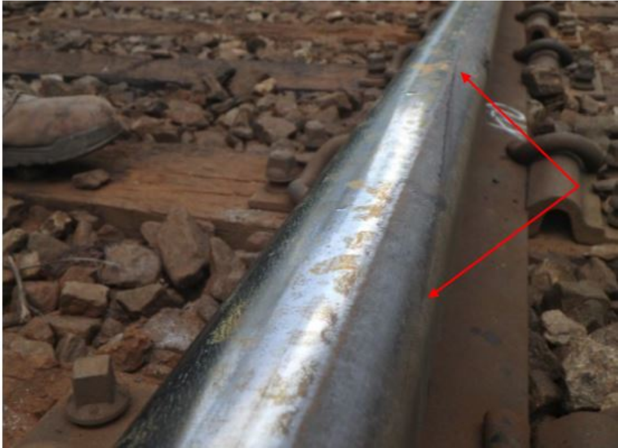
Figure 8. Flange mark at point of departure of FWTX 620111 (35th car).
