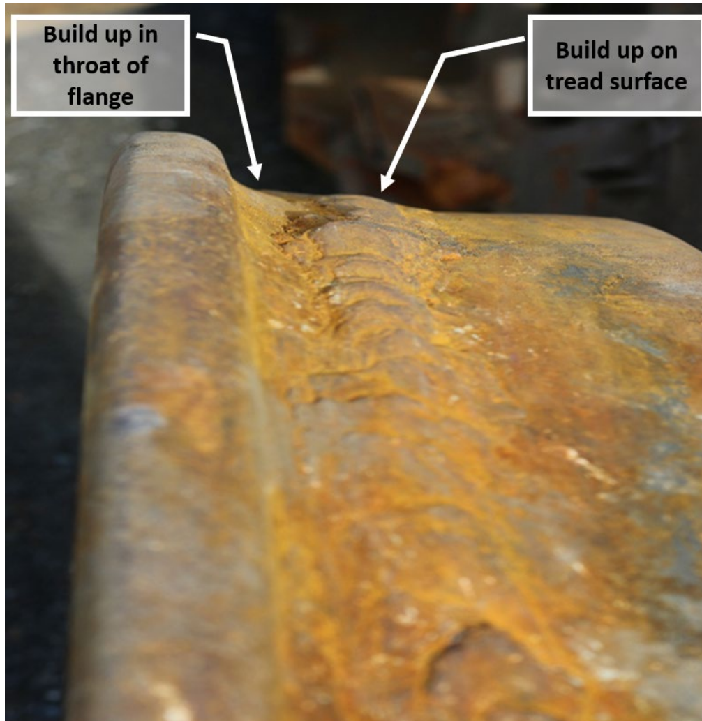
Figure 6. Closeup of wheel tread surface showing tread buildup on wheel of the 35th car.
