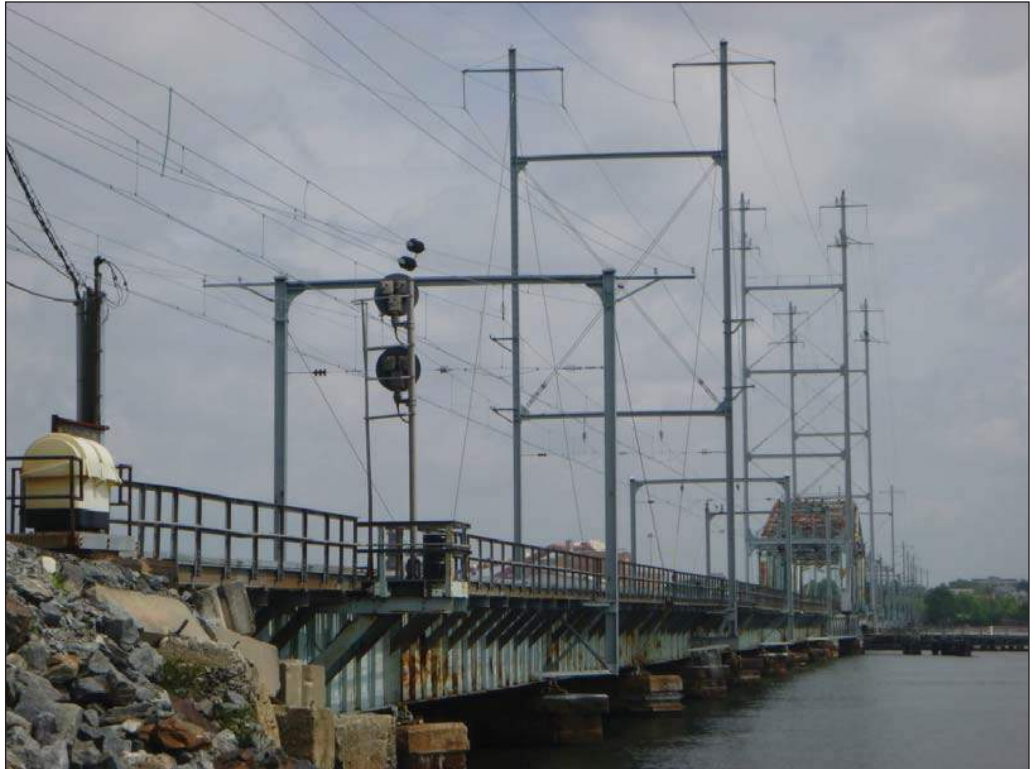
Raritan River Draw Bridge (Map ID 1) and Overhead Contact System (Map ID 2)
